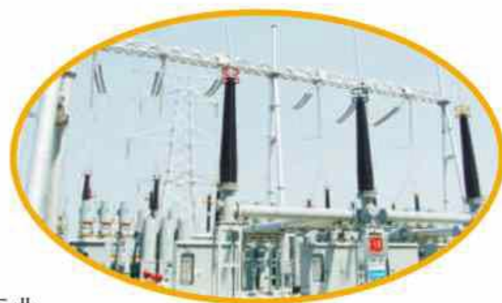
能源/电力行业 Energy/Electric power
